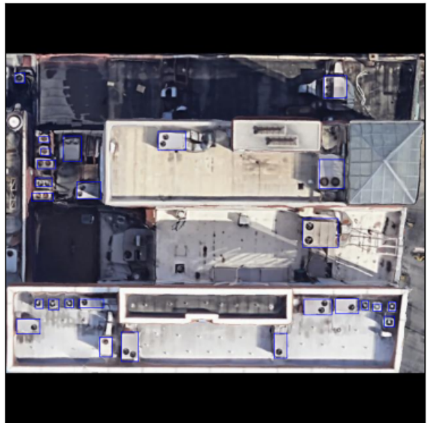
Figure 4. An example of a rooftop containing many RTUs (outlined in blue) of varying type and dimension.
